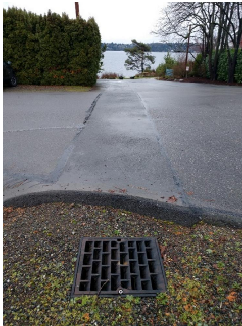
Photo N9 – Facing west along SE 28 th St approximately 95 feet west of Photo N8 at southeast corner of the intersection of SE 28 th St and 60 th Ave SE. Runoff is conveyed via this catch basin on the south side of the street toward Lake Washington.
